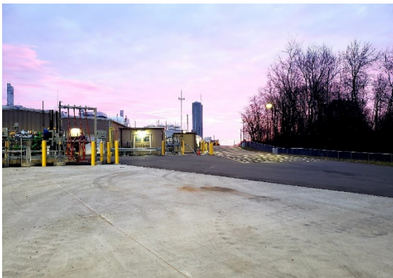
The offloading station was part of a larger project to process the County's landfill biogas for pipeline injection.
