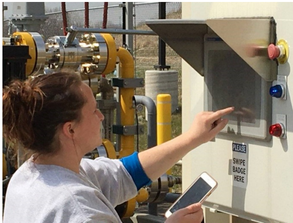
Dane County Department of Waste & Renewables engineer, Ali Rathsack, finalizes programming the controls at the offloading station. County staff and industry partners worked diligently to demonstrate that the proper controls and protocols were in place to meet the rigorous requirements of the U.S. EPA's renewable fuel standards.
